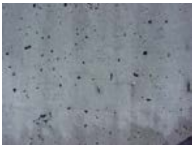
Figure 1: Example of voids on the surface of a concrete tilt-up panel.
