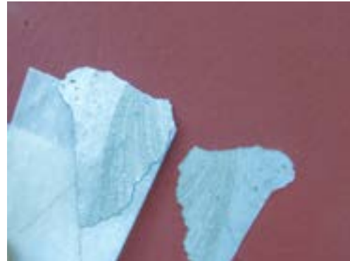
Figure 3: Sacking failure on tilt-up panel, verified using ASTM D3359 Test Method A – X-Cut Tape Test.
